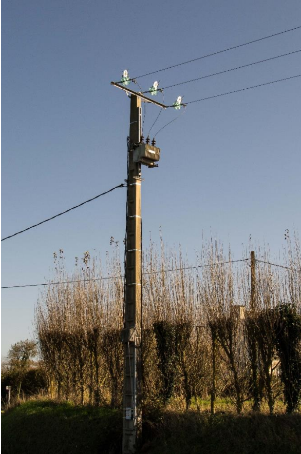
Transformer 20 kV/220 V
